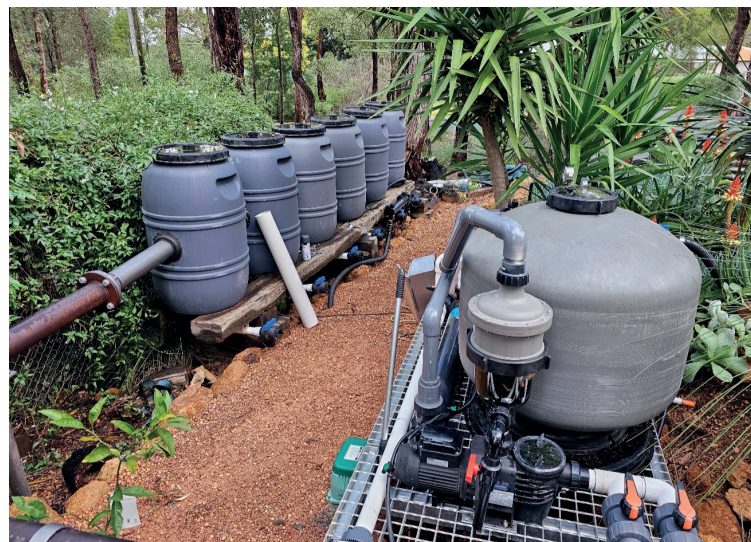
Figure 1. Filtration equipment for the 20 kL pond.
